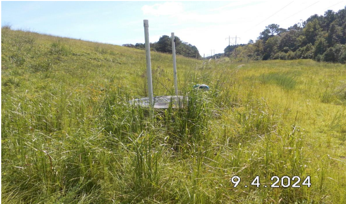
Photograph AA – Overgrown Area along Right-of-Way
