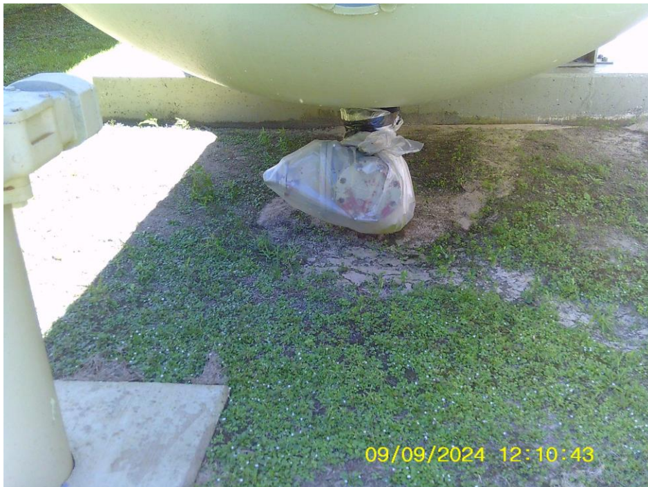
Photograph O - Surge Tank Drain Piping
