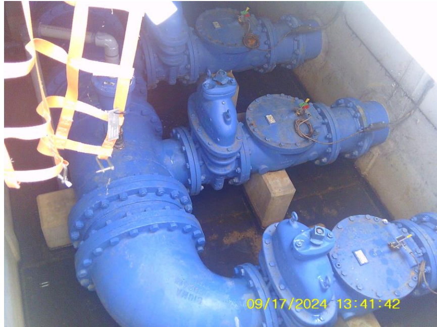
Photograph U –Transfer Pump Station Valve Vault
