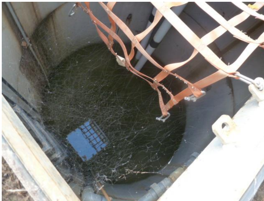
Photograph DD- NPDES Chemical Injection Vault
