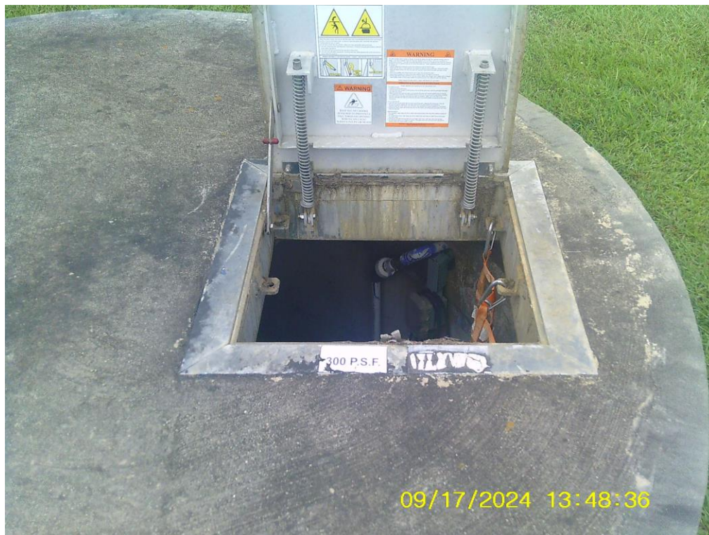
Photograph V- Transfer Pump Station Check Valve Vault
