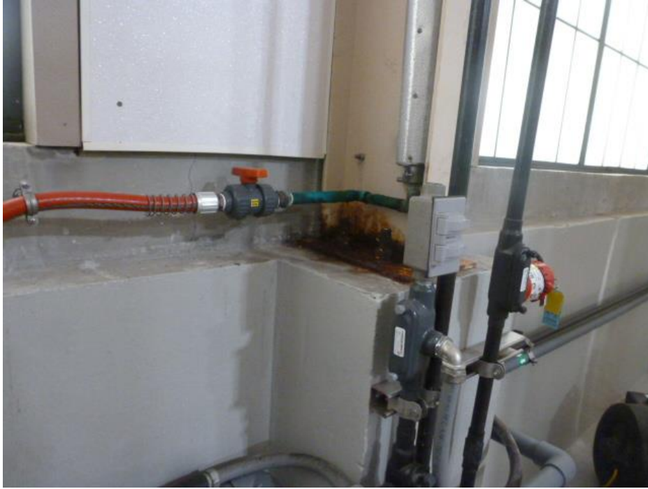
Photograph Y- Chemical Building Interior Piping Leak
