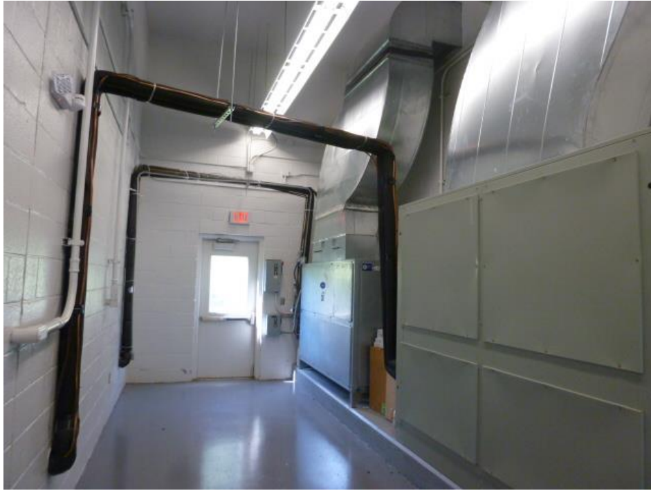
Photograph H - Electrical HVAC Room
