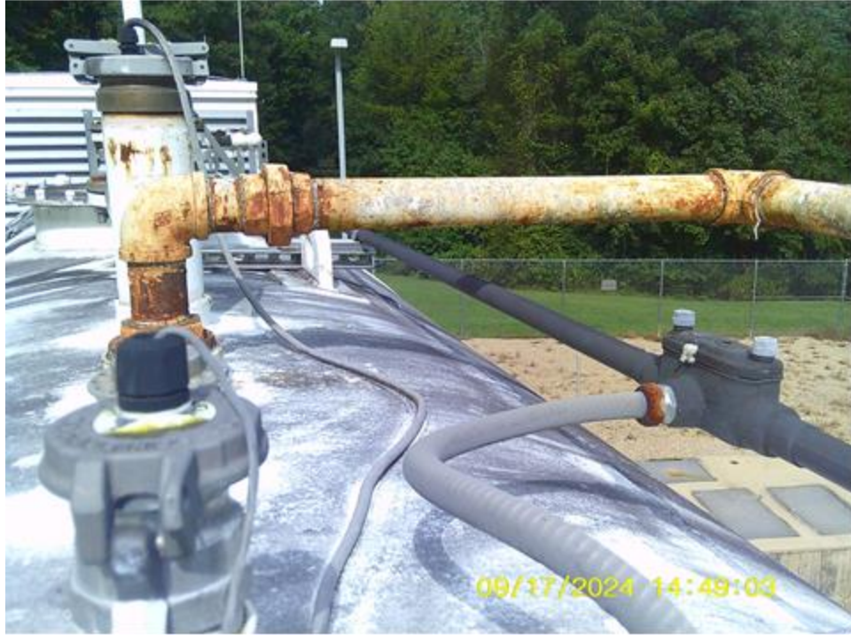
Photograph I – Diesel Storage Fuel Piping
