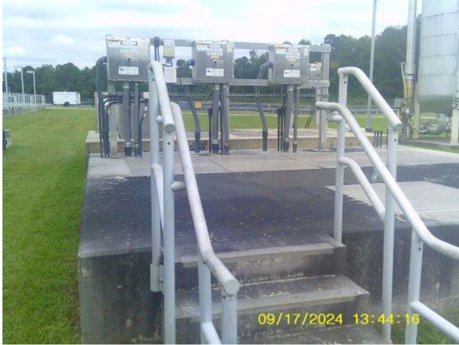
Photograph S –Transfer Pump Station
