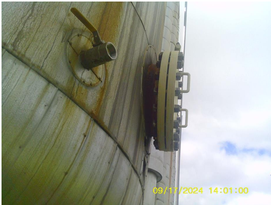
Photograph X- GAC Filter Manway Corrosion
