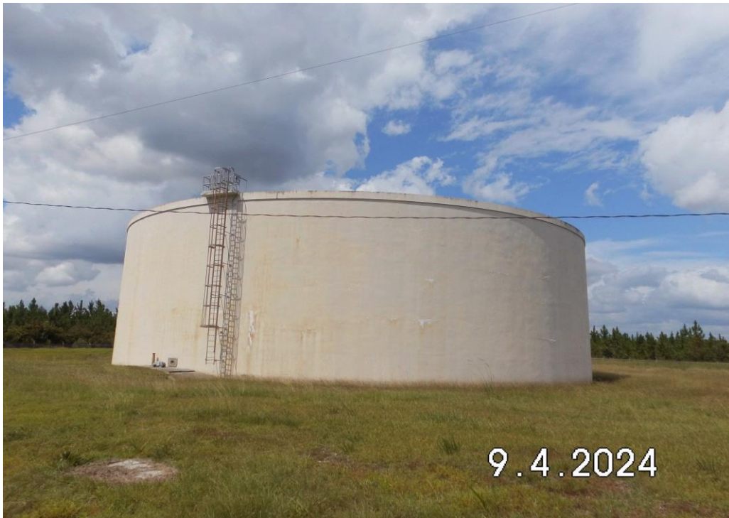
Photograph JJ- 3 Million Gallon Ground Storage Tank
