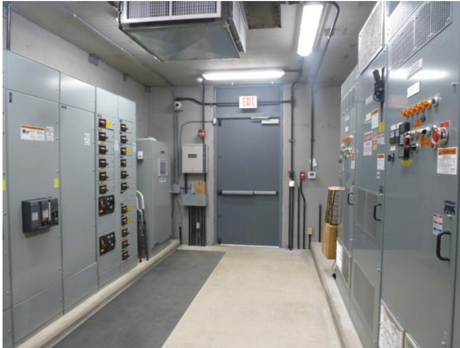
Photograph G – Pump Station Electrical Room
