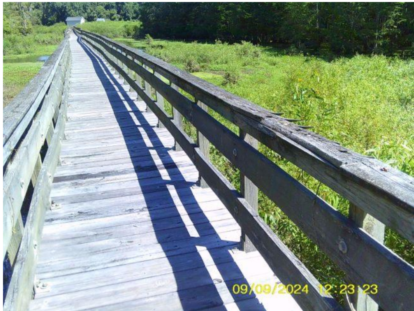
Photograph T – Pier Rotten Boards
