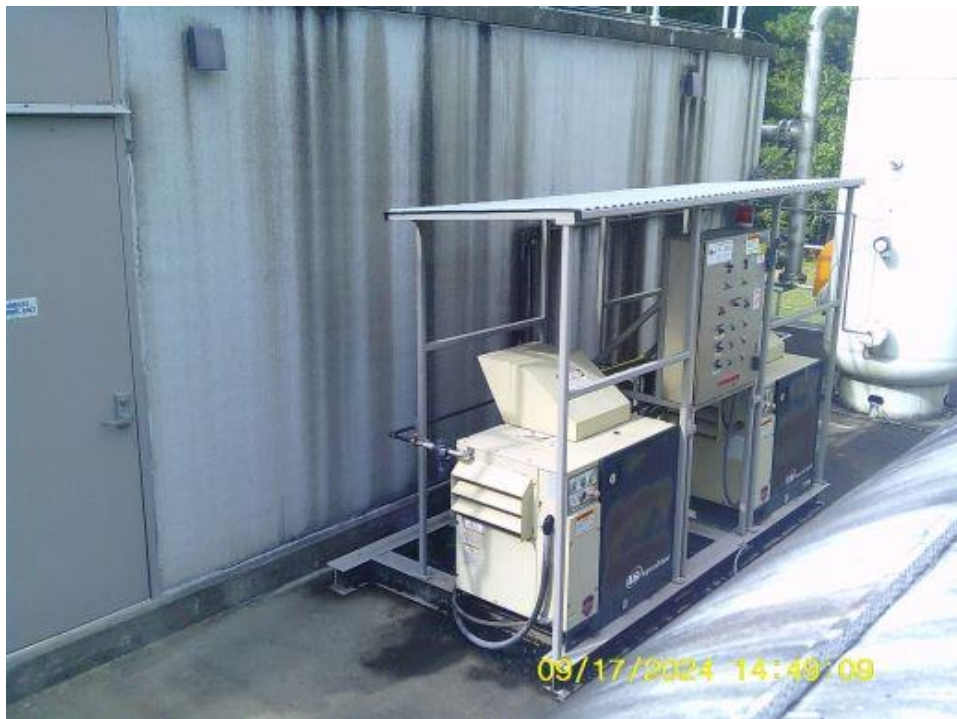
Photograph L – Air Backwash Compressor
