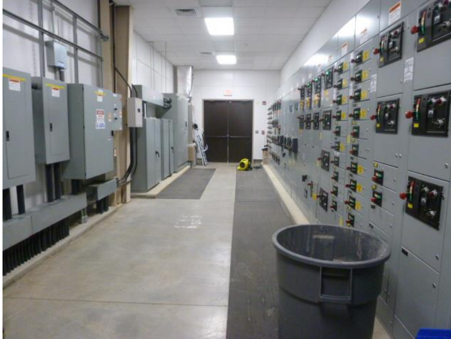
Photograph AA- Chemical Building Electrical Room
