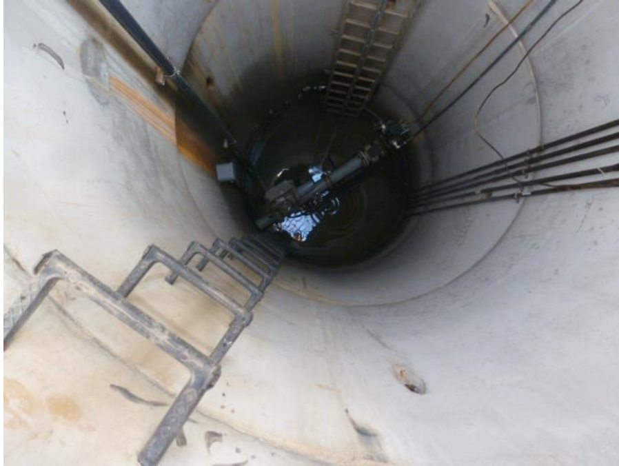
Photograph CC- NPDES Compliance Wet Well
