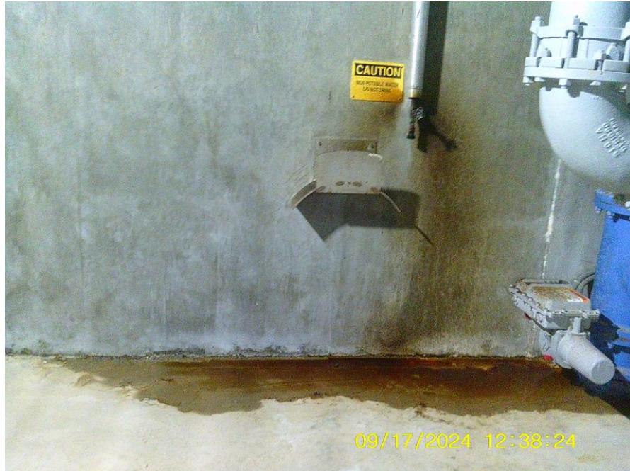
Photograph R – Filter Gallery Piping Leaks
