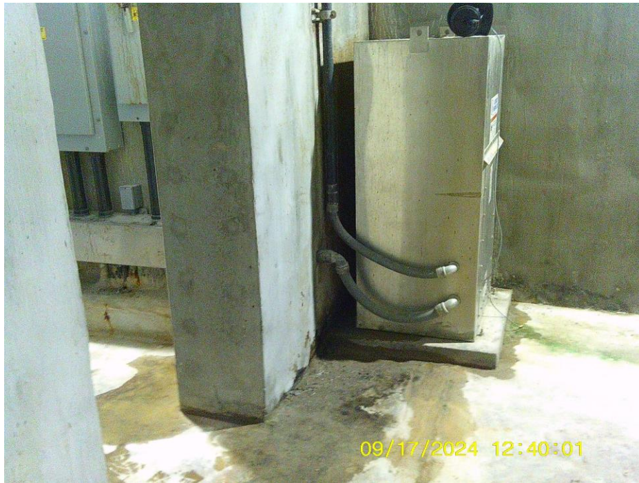
Photograph Q – Filter Gallery Wall Leaks
