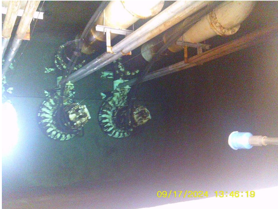
Photograph T –Transfer Pump Station
