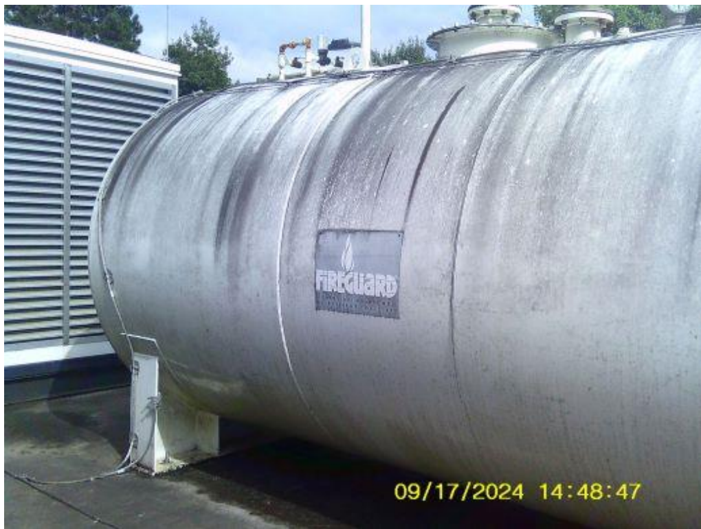
Photograph H – Diesel Storage
