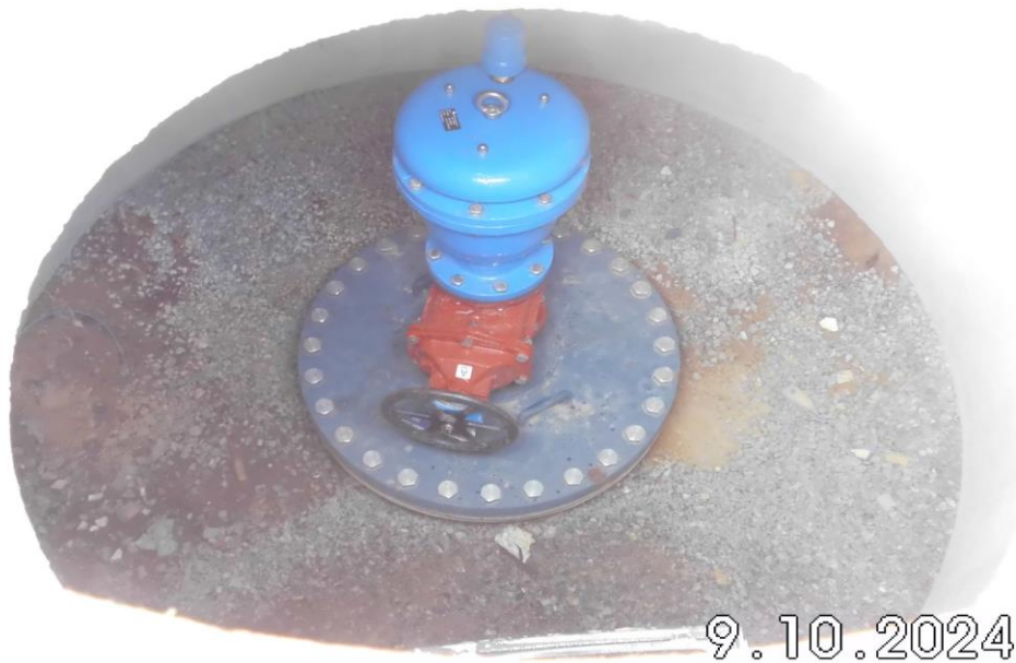
Photograph DD – Old ARV on 48" RWM and New ARV on 54" RWM
