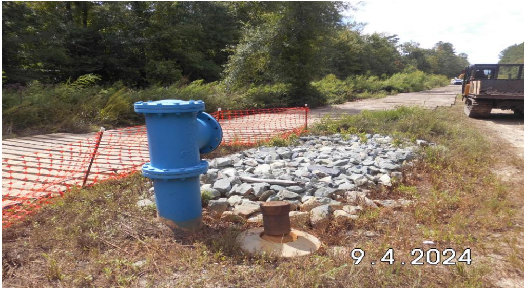
Photograph GG- Old Blow-off on 48" RWM and new Blow-off on 54" RWM
