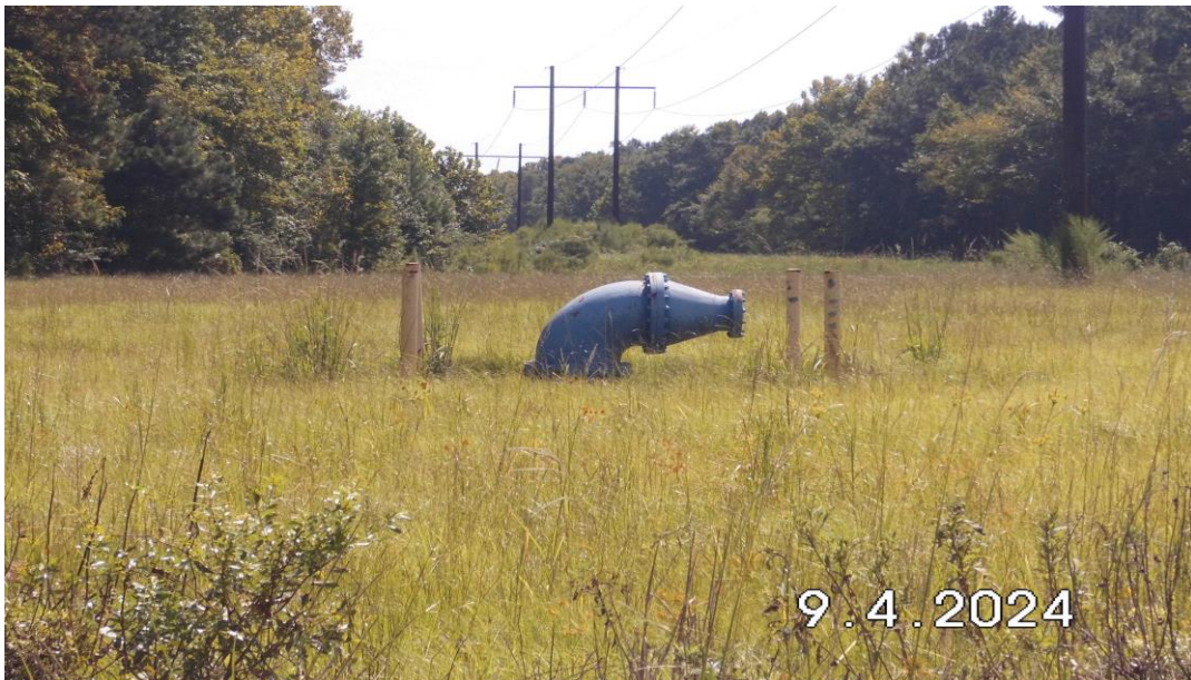
Photograph EE- Emergency Intake Pipe Adjacent to Pond behind DAK
