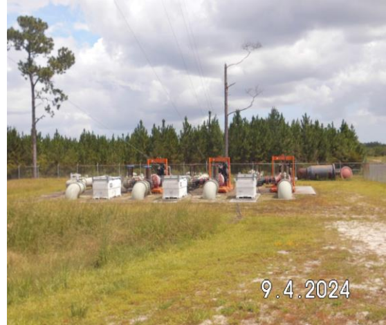
Interim Raw Water Booster Pump Station
