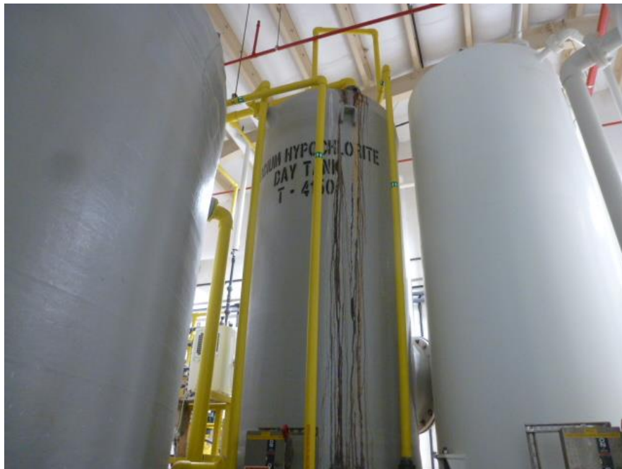
Photograph Z- Chemical Building Chlorine Tank Leak
