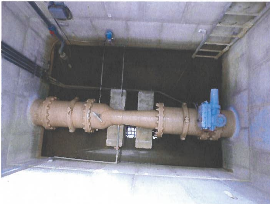
Photograph K – Influent Flow Meter Vault
