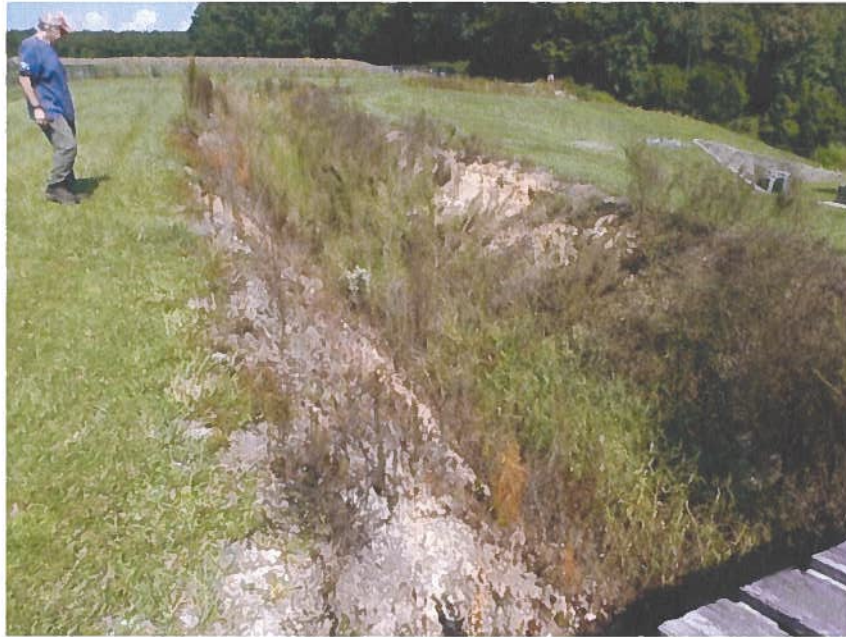
Photograph H – Upper Ditch Erosion
