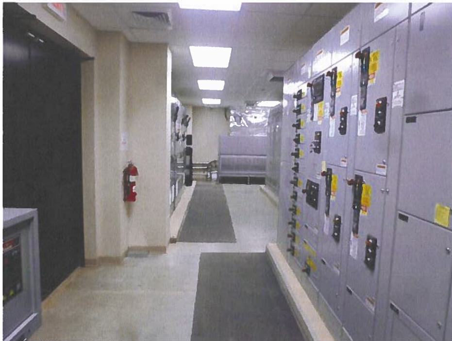
Photograph W- Administration Building Electrical Room
