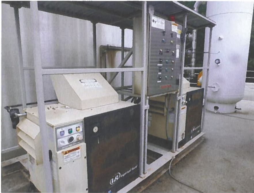
Photograph J -Raw Water Pump Station Backwash Compressor
