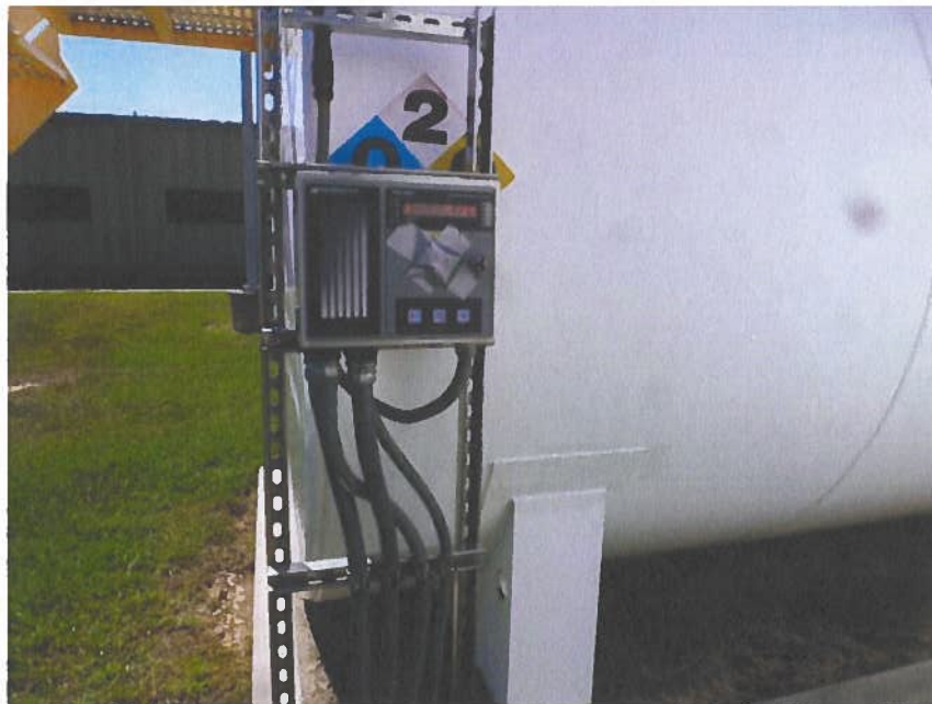
Photograph Y- Facility Generator Diesel Tank Leak/Level Panel
