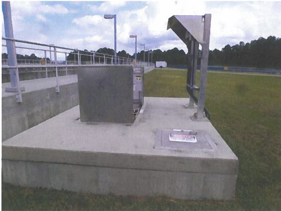
Photograph L – Influent Flow Meter Vault
