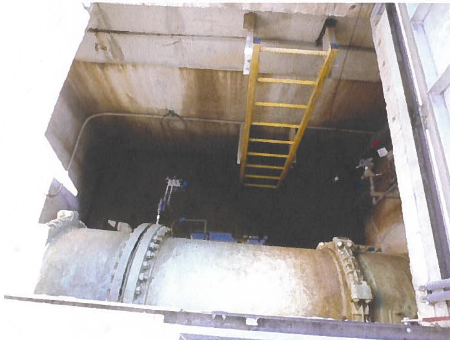
Photograph E – Raw Water Flow Meter Vault
