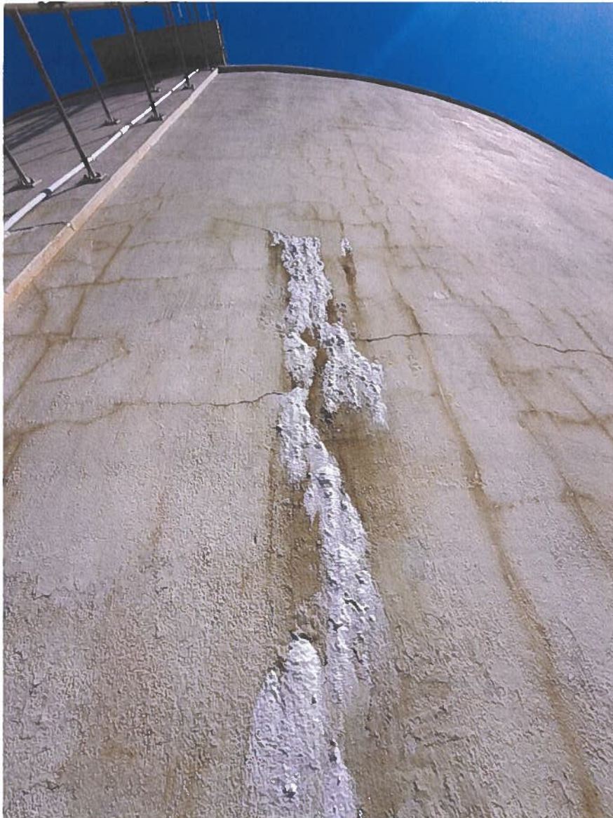
Photograph JJ- 3 Million Gallon Ground Storage Tank Calcification
