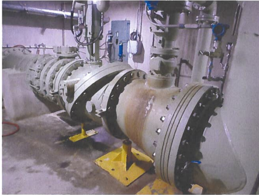
Photograph B – Check Valve on Pump #4 Dash Pot Leaking
