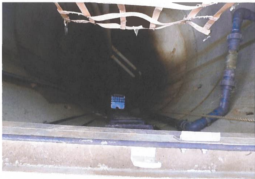
Photograph AA- NPDES Compliance Chemical Injection Vault
