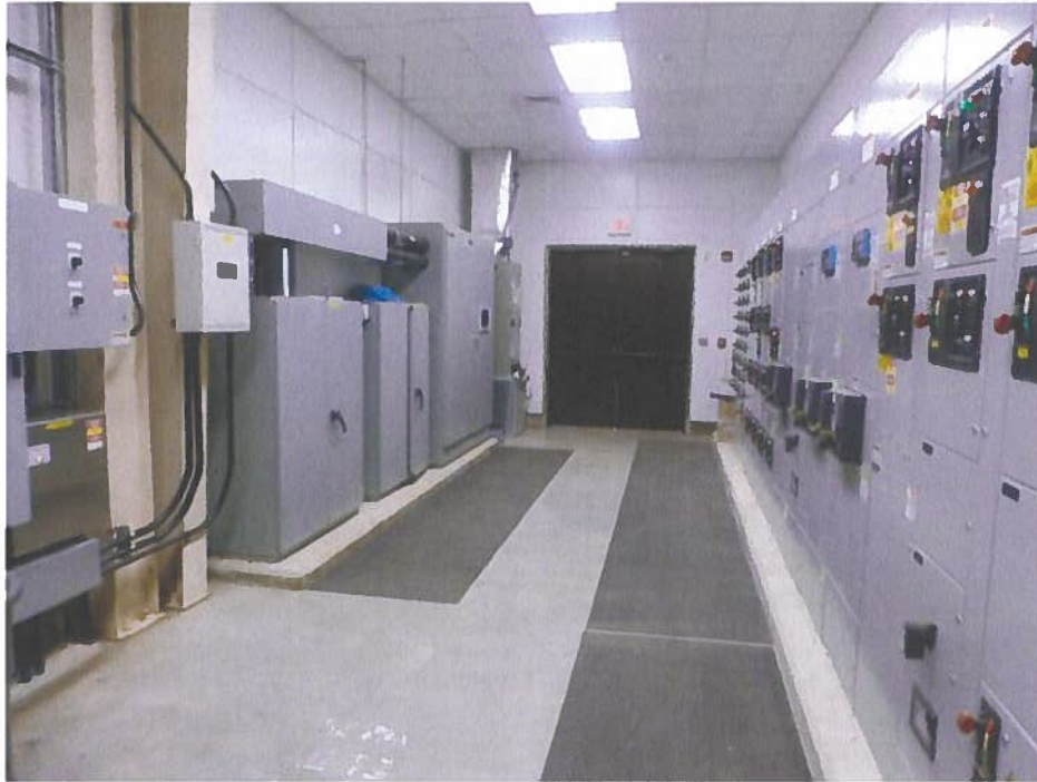
Photograph V- Chemical Building Electrical Room
