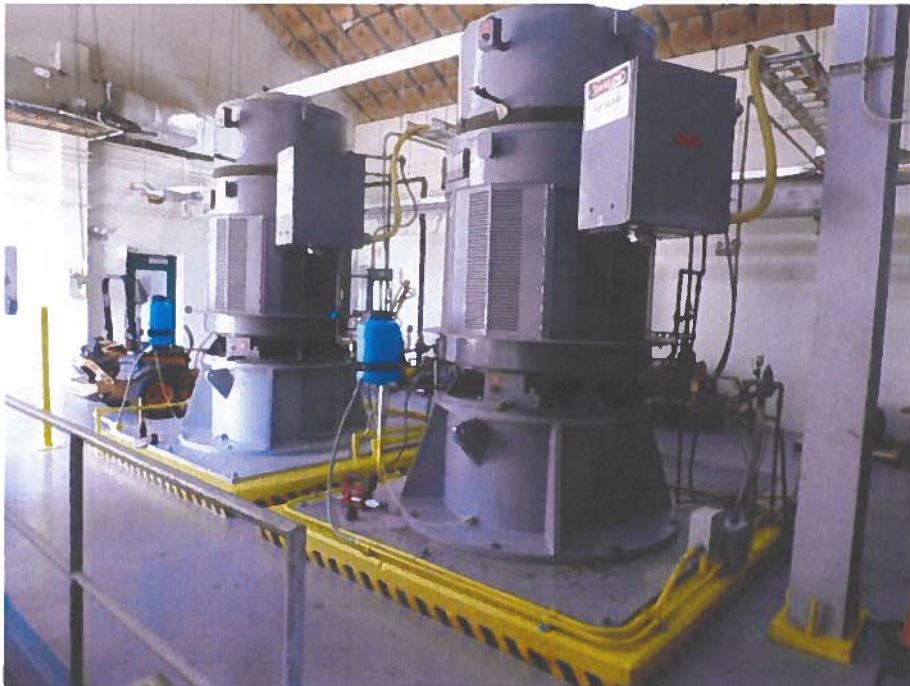
Photograph A – Pump #4 and #5
