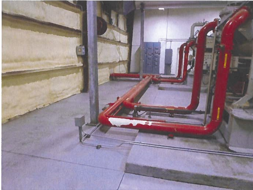
Photograph R – Generator Coolant Piping
