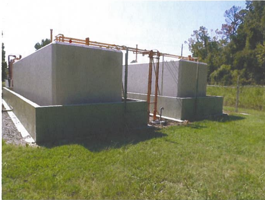
Photograph F –Generator Diesel Storage Tanks
