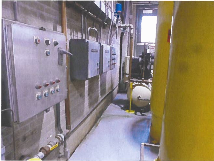
Photograph J - Surge Tank Controls
