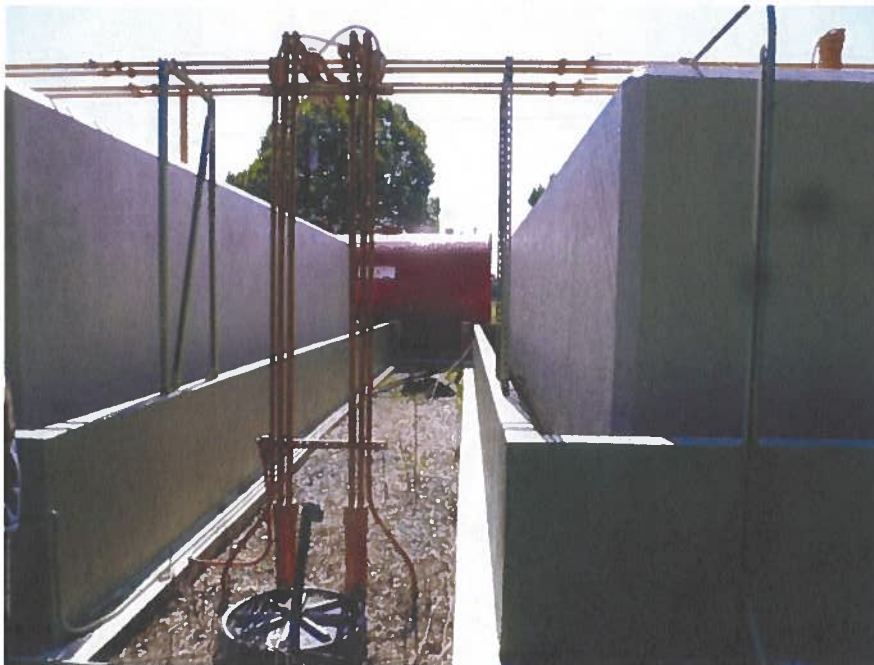
Photograph G – Generator Fuel Transfer/Feed Piping
