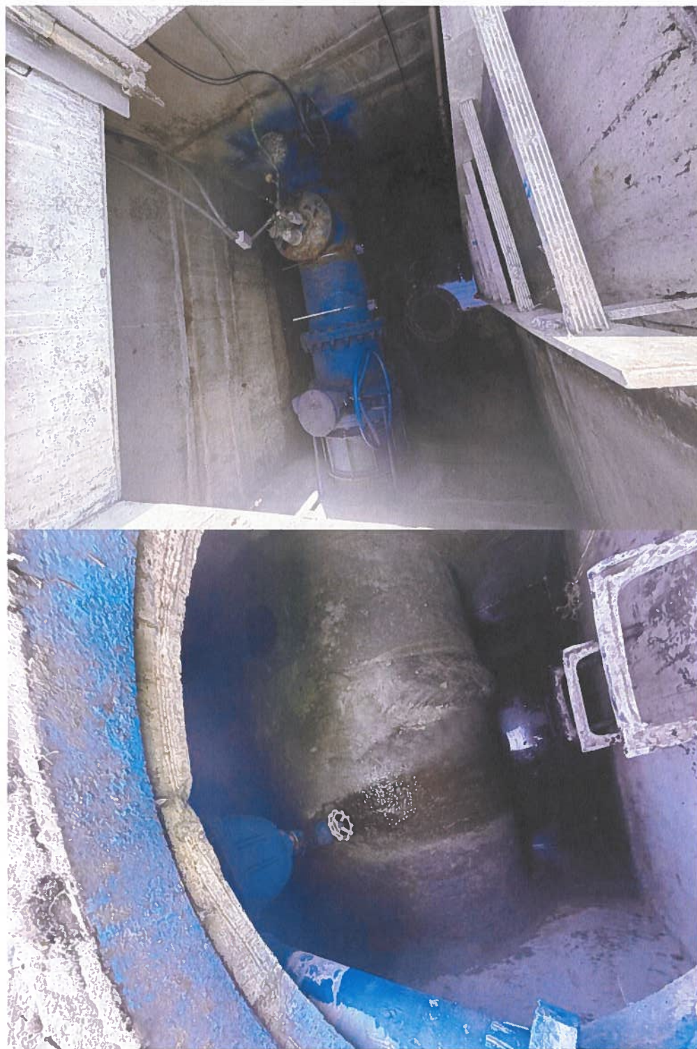
Photograph CC – Leaking ARV at Praxair
