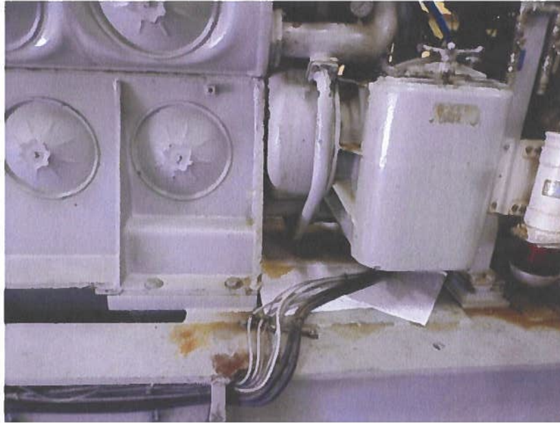
Photograph M – Generator #2 Coolant Leak
