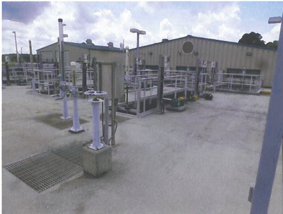
Photograph N – Flocculation Basin and Filter Area
