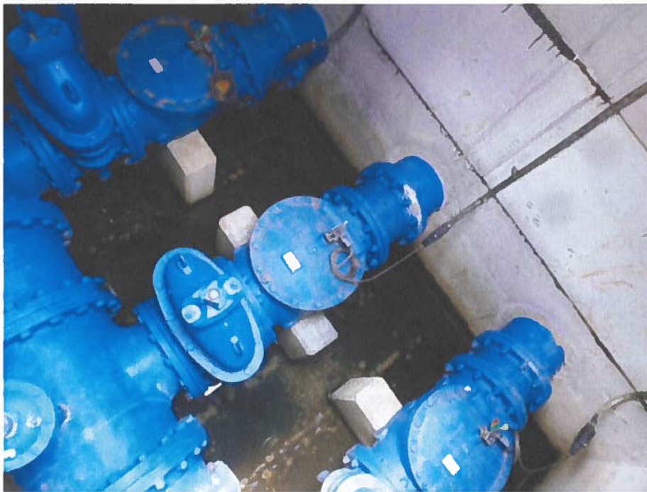
Photograph Q –Transfer Pump Station Valve Vault
