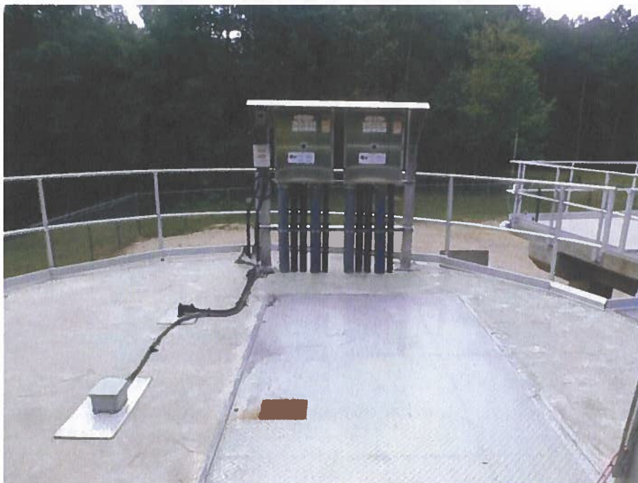
Photograph E – Intake Wet Well
