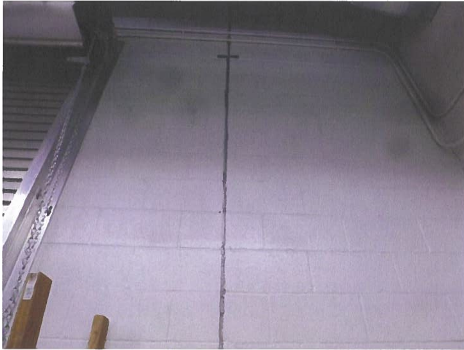
Photograph D – Masonry Control Joint in Electrical Room
