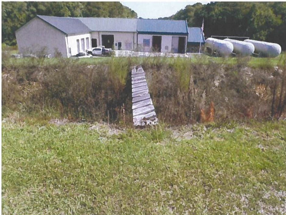
Photograph I –Failing Protective Bridge
