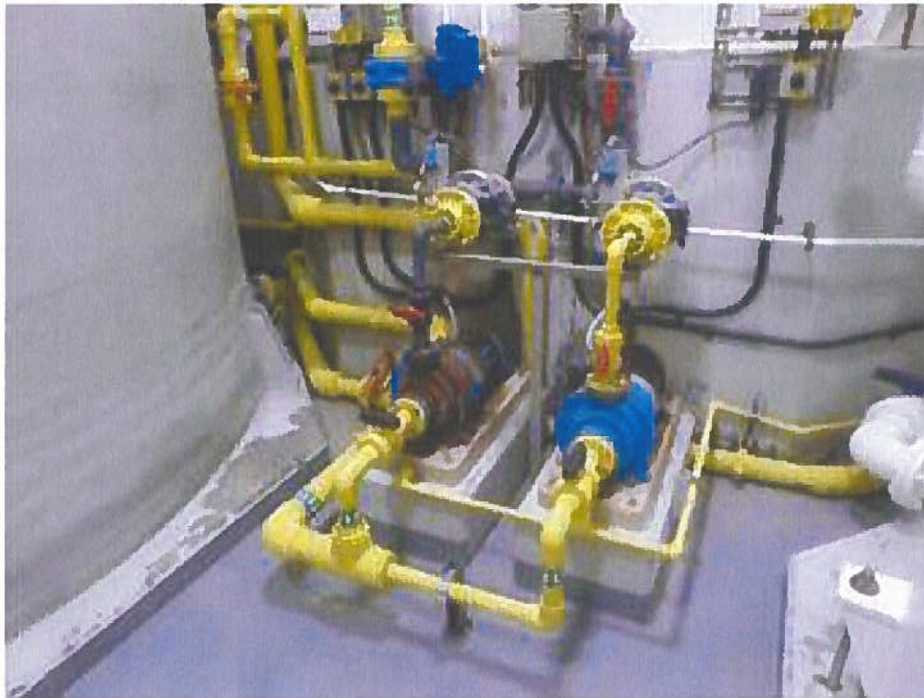
Photograph T - Chlorine Transfer Pump
