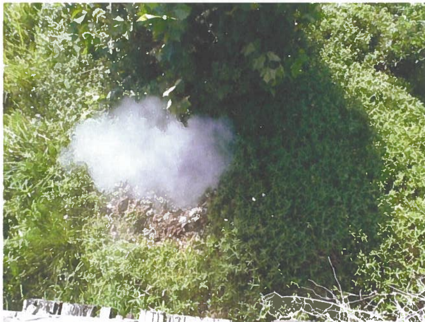
Photograph O –Old Backwash System Leak
