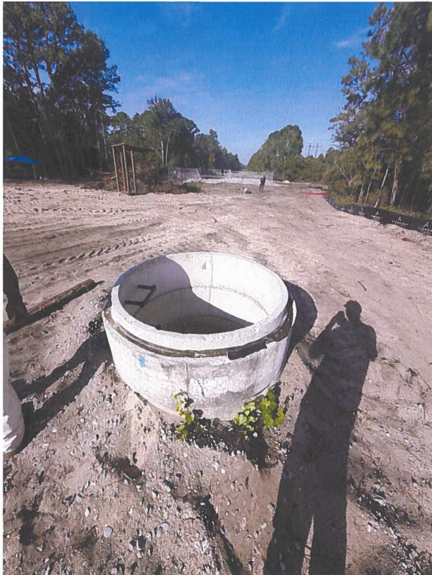
Photograph AA – Structure Damage during construction of 54" RWM
