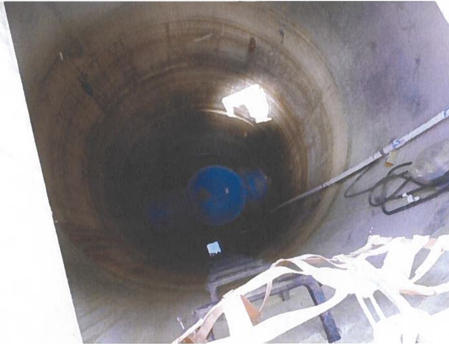
Photograph R –Transfer Pump Station Check Valve Vault
