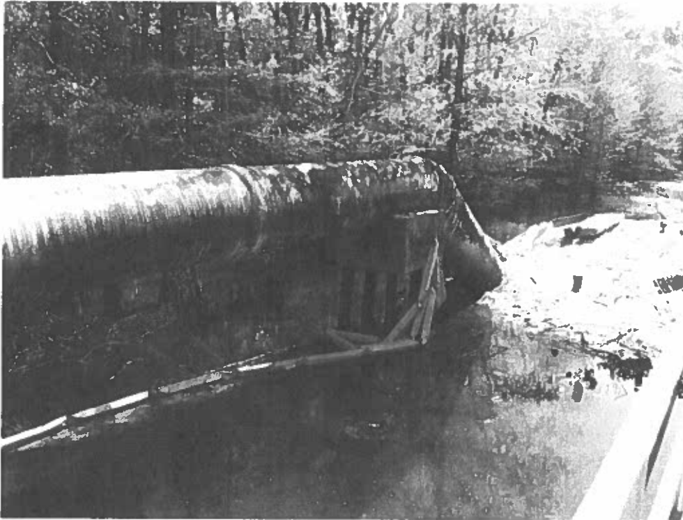
1. View Looking East at Pipe Support #1 & where Access Road Intersects w/ South/East Bank of Livingston Creek.
