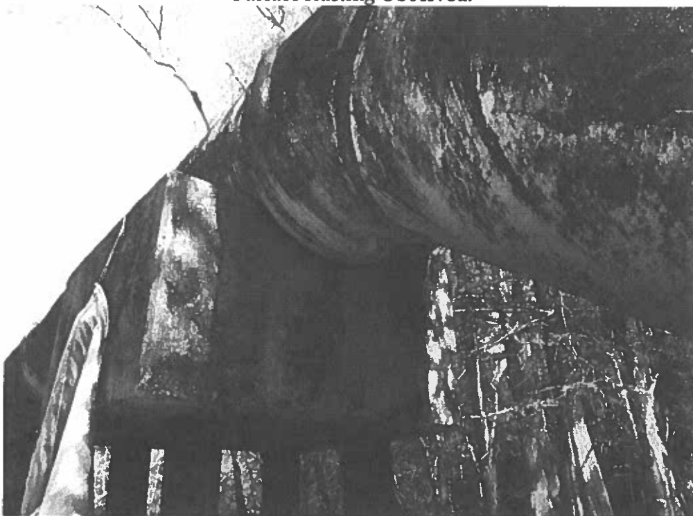
12. View Looking at the Underside of the Pipe Joint South of Pipe Support #1 & the Exposed and Cracked Grout.
