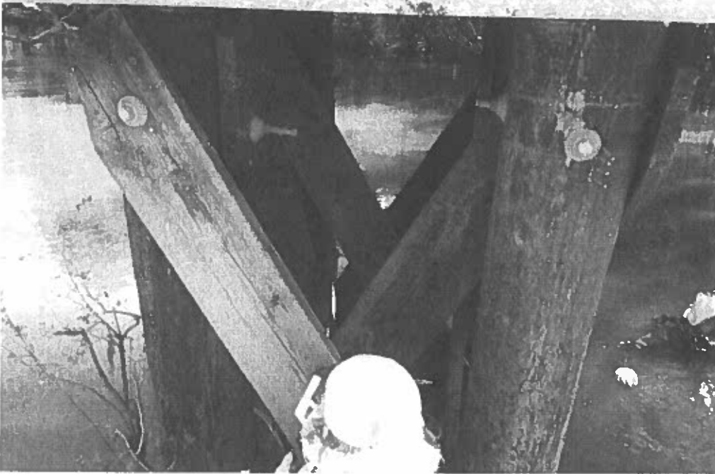
11. Close-Up View of Timber Pile / Bracing Fastener Connection Assemblies & the Surface Rusting Observed.
