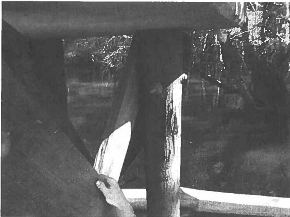
6. Close-Up View of South Face of the Southeast Pile (P3) of Pipe Support #2 where Surface Peeling was Observed.
