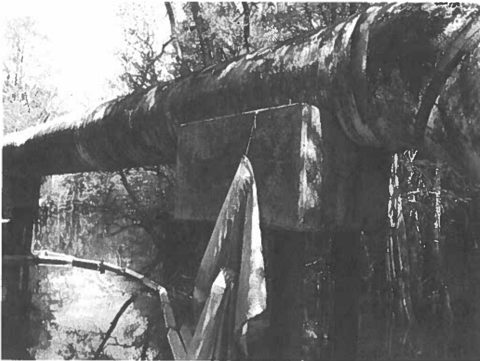
5. View Looking at the Southwest Pile (P4) of Pipe Support #1 where Minor Split Lines in the Pile were Observed on the South Face of the Pile.
